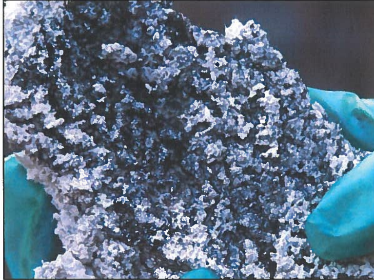
Mold growing on a piece of ceiling tile.
