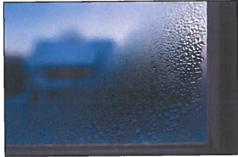
Condensation on the inside of a windowpane.
